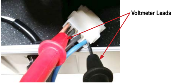
Testing Compressor Voltage
